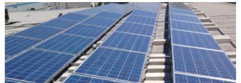
Figure 28: Plot One solar panels
